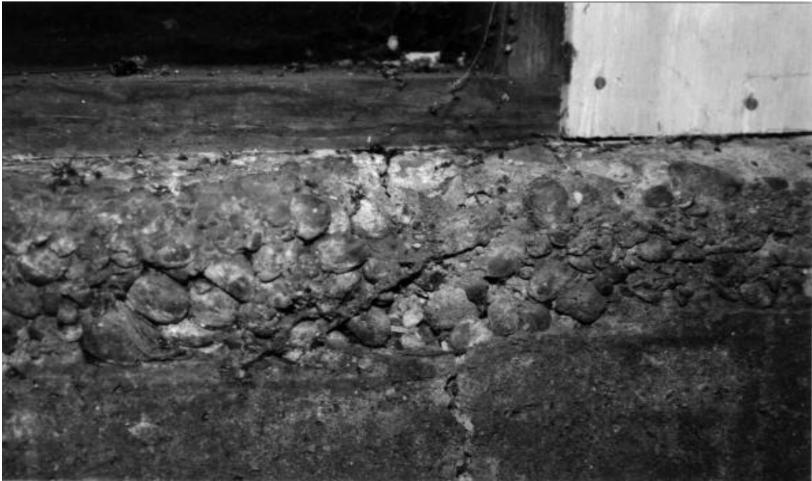
Figure 7. This foundation wall shows signs of deterioration and cracking. Problems with the foundation may not be identified until installation of the retrofit anchor bolts. (Photo by Gary Milici, RetroFitters).
