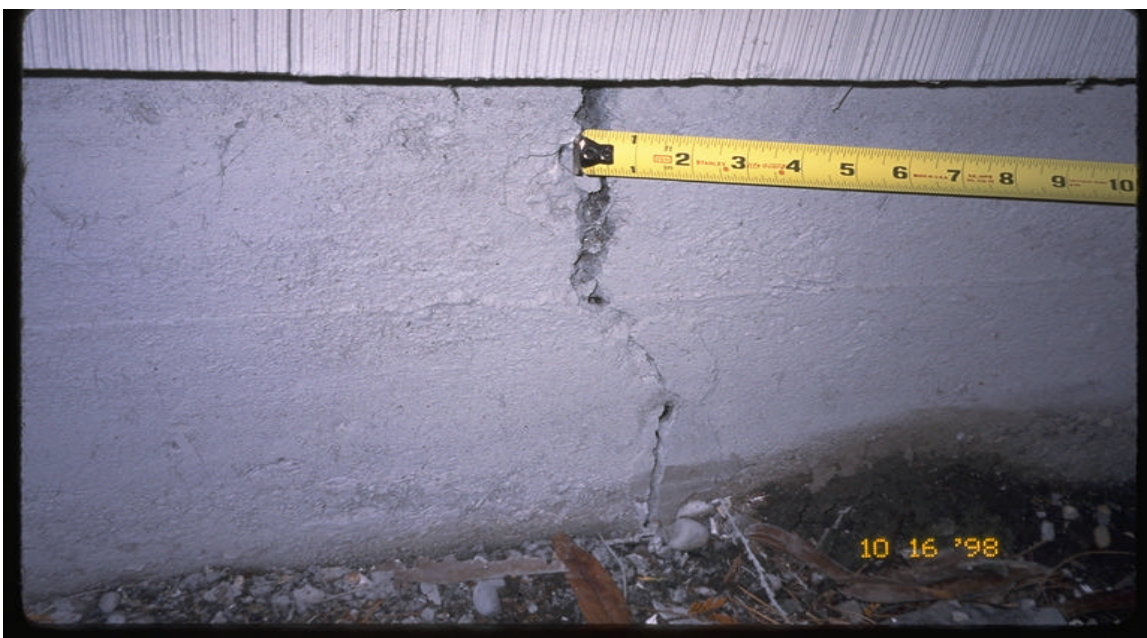
Figure 6 The foundation should be in good conditions. This ½ inch crack may need to be repaired before completing the earthquake retrofit. (Photo by Linda Noson, AGRA Earth & Environmental)
