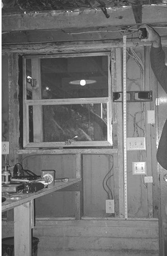
Figure 9 The height of the pony wall is measured from the bottom of the sill plate to the top of the double plate. A home with a pony wall over 4 feet like this one, which is about 5 feet, does not qualify to use the Standard Home Earthquake Retrofit Plan. (Photo by Linda Noson, AGRA Earth & Environmental)
